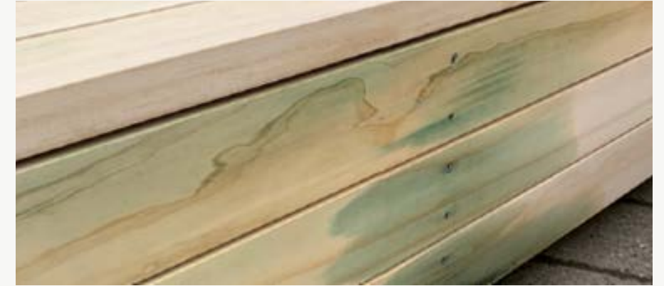
Wicking of pressure treated softwood framing chemicals through Accoya
